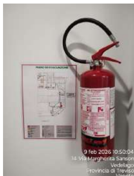
Fire extinguisher and floor plans.jpeg
